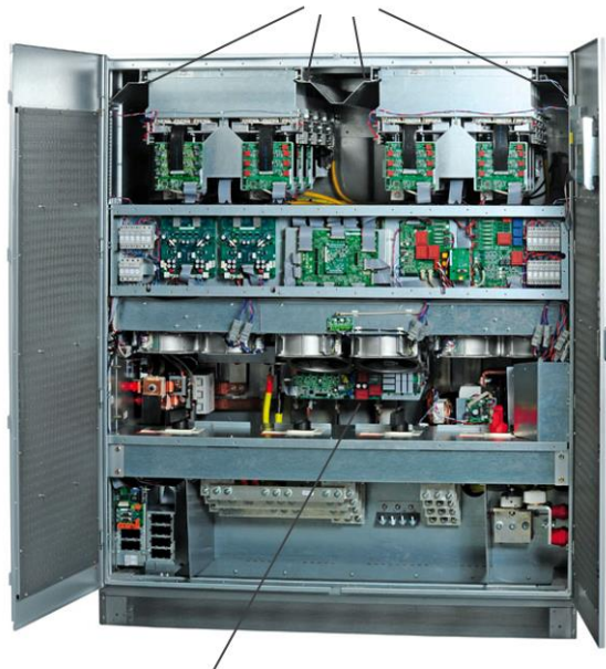
Capacitors are mounted on withdrawable rails
